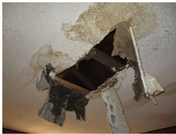
Roof and interior damage (2) cabins
