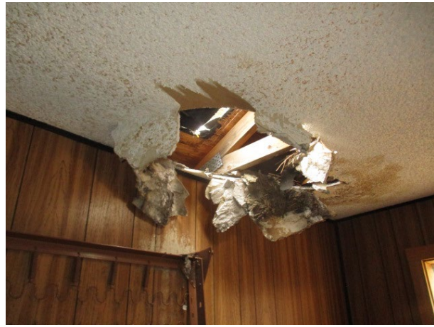
Second cabin ceiling damage
