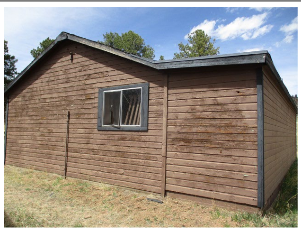
Exterior peeling paint, broken windows and screens
