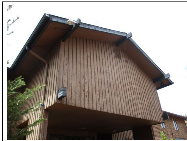
Front of building peeling paint
