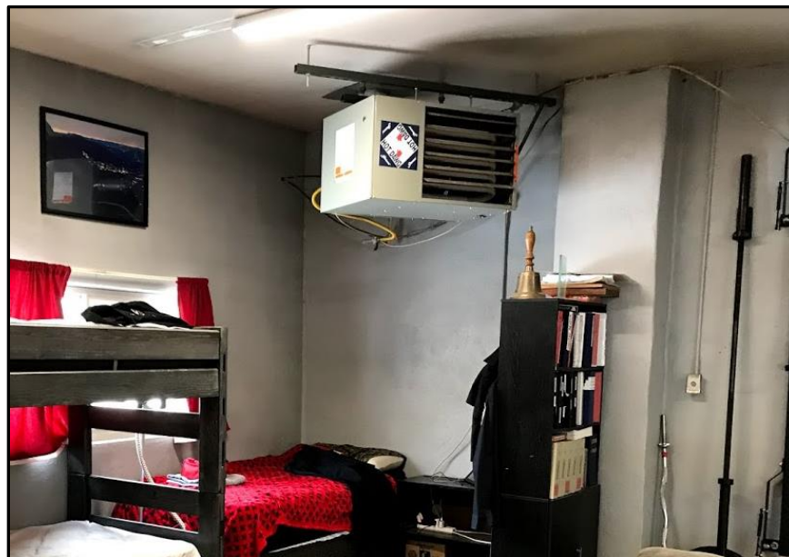
Figure 15: Overhead Heater in Sleeping Area
